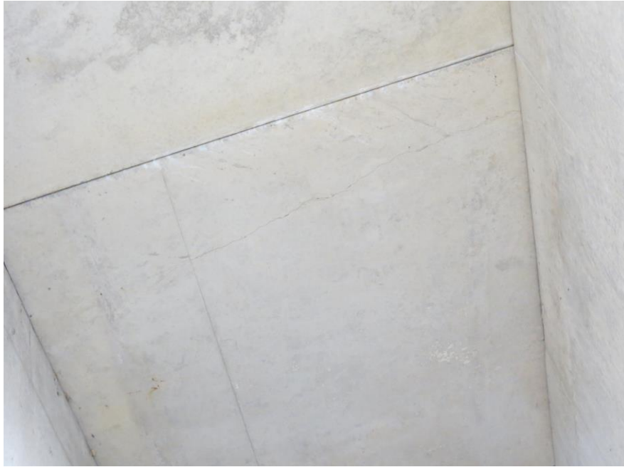
DECK PANEL BAY "A" ABUT. #2 W/ CRACK
