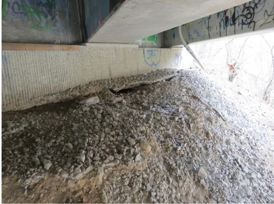
SETTLEMENT AT ABUTMENT #2
