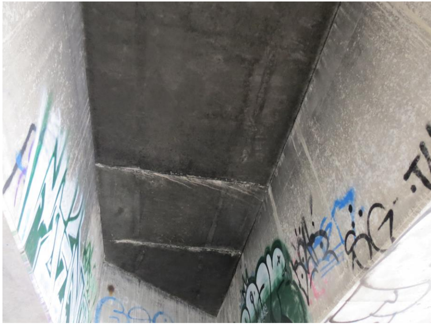
DECK PANEL BAY "B" ABUT. #2 W/ FIRE DAMAGE
