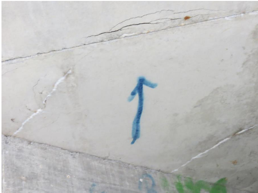
DECK PANEL BAY "D" ABUT.#2 W/ CRACKS
