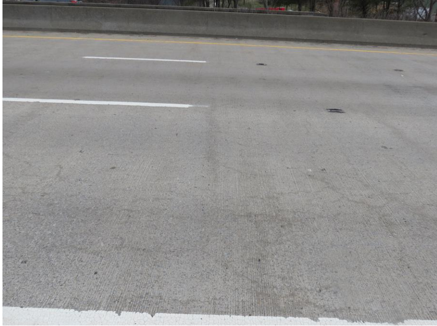
WEARING SURFACE SP. #2 W/ CRACKS
